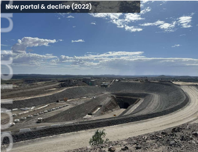
750,000tpa capacity processing facility
